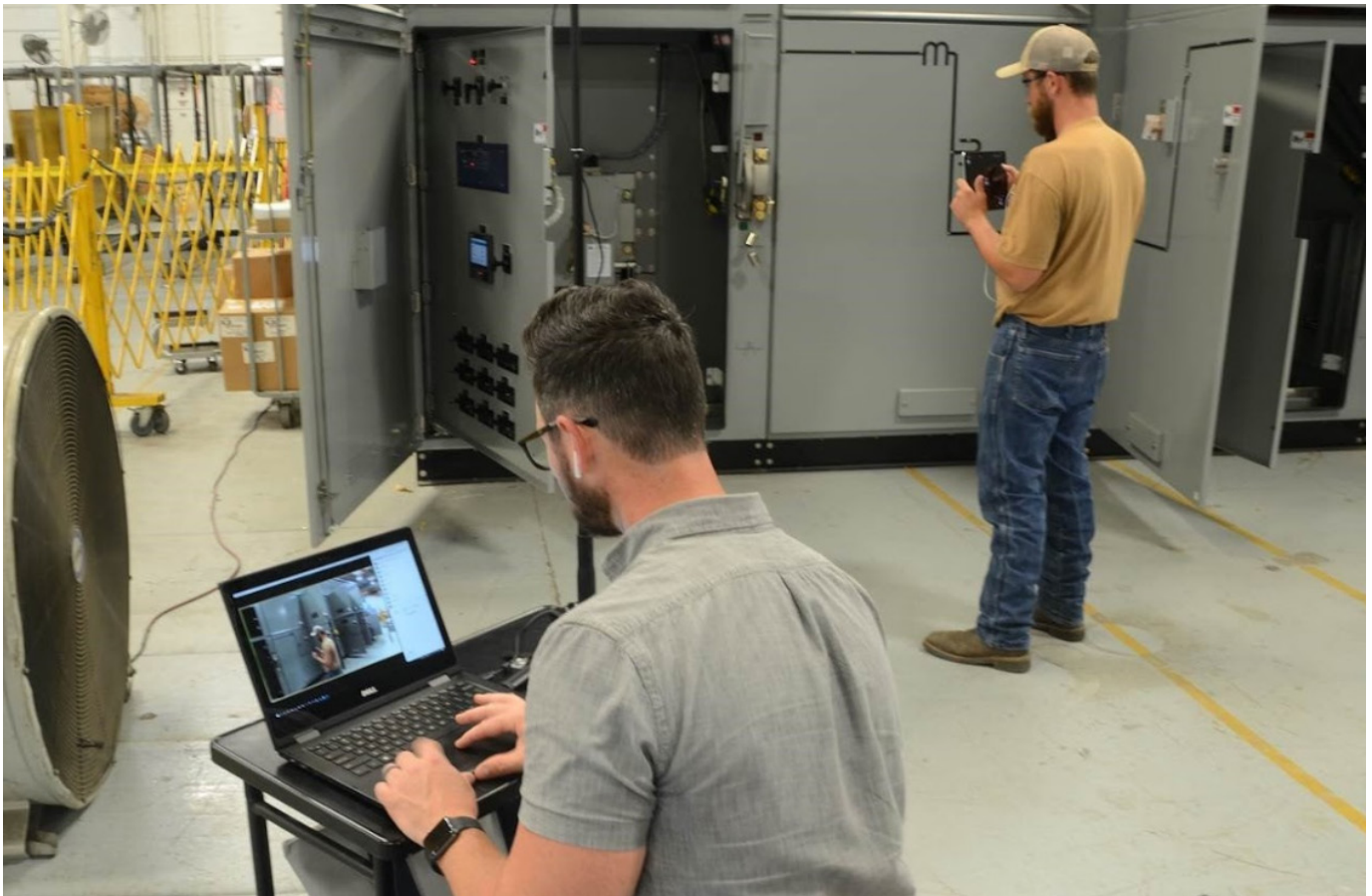
Electro-Mechanical LLC on Goodson Street was founded in 1958 and is one of America's largest manufacturers of power distribution components.
